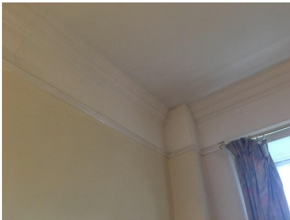
Fig. 31 Overpainted stucco cornice, with services riser in corner.
