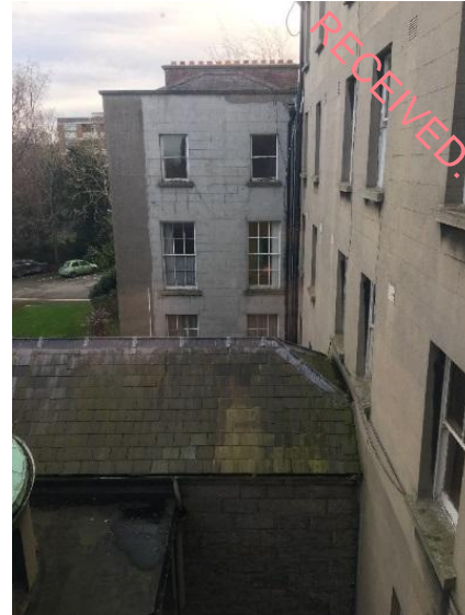
Fig. 26 Part of rear (west) elevation, with uppermost level added, and in context with its higher rear extension.
